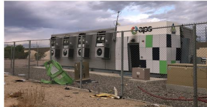
ESS System Explosion in AZ
